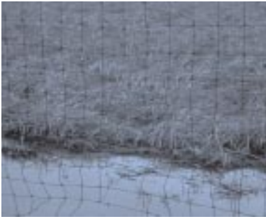
Airport fence with hole
